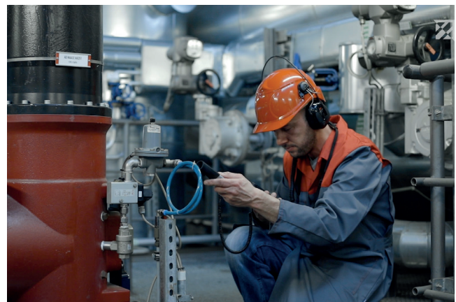
Detection of leaks on a compressed air line with the SONAPHONE
